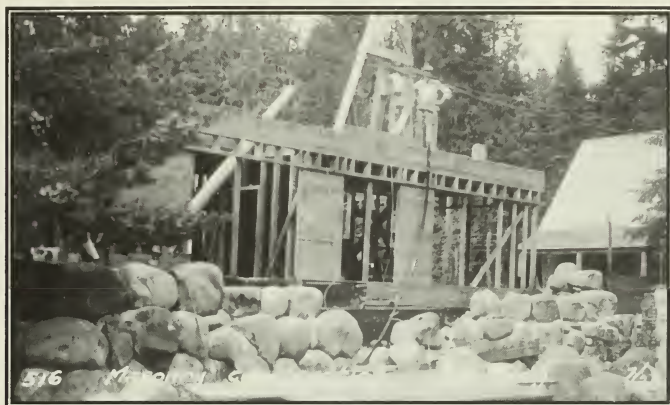
Construction on the new Administration Building at Longmire began on May 14, 1928. The Park wanted the building to be "the show place of the Administrative group. A great deal of care was taken with the plans and construction." (Park Structures Collection)
